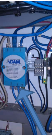
A picture of: Commutations main interface for all equipment inside bldg 8760 ORNL-SNS.
